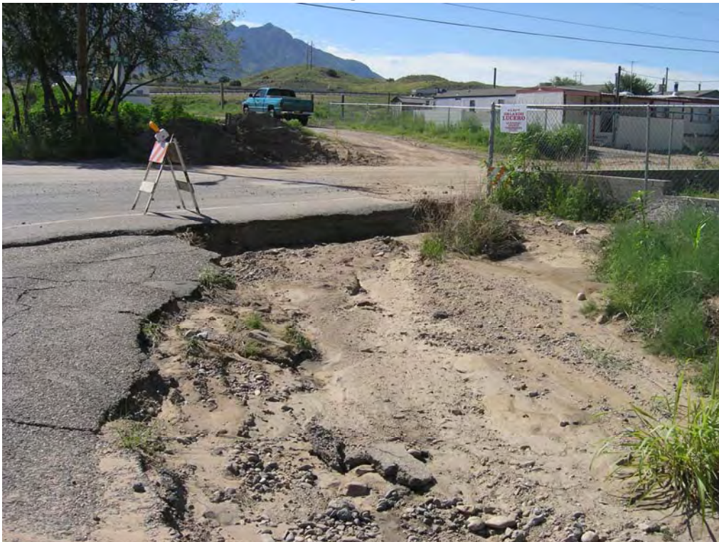
Erosion due to high waters crossing South Hill Rd. at Avenida Bernalillo
