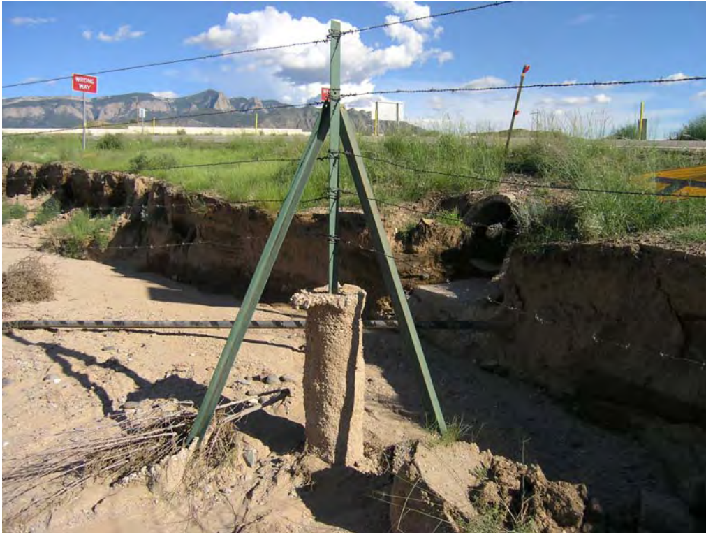
Ongoing erosion conditions at I-25 and Avenida Bernalillo
