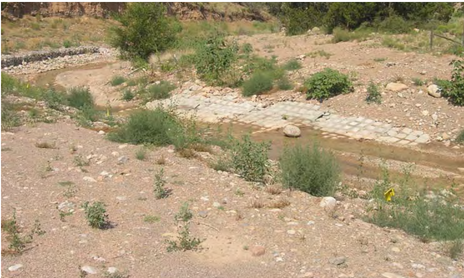
Concrete erosion control blanket over utility pipelines just west of Camino de las Huertas between Cedar Creek Rd. and Windmill Trail
