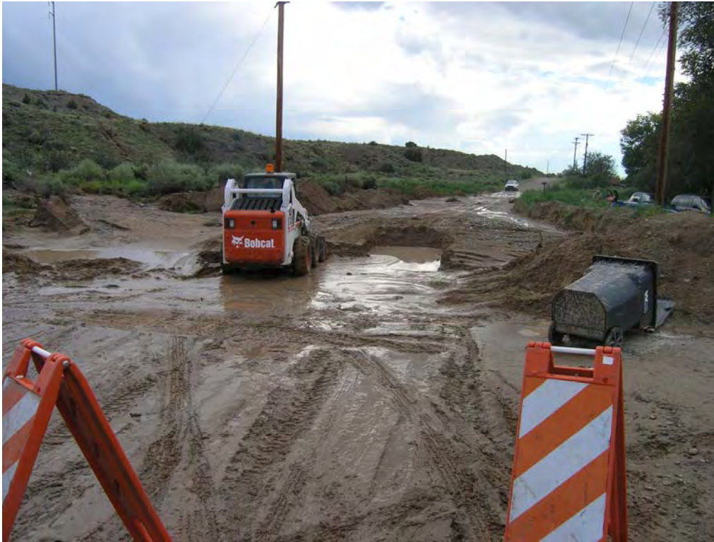
Sediment deposition on South Hill Rd.
