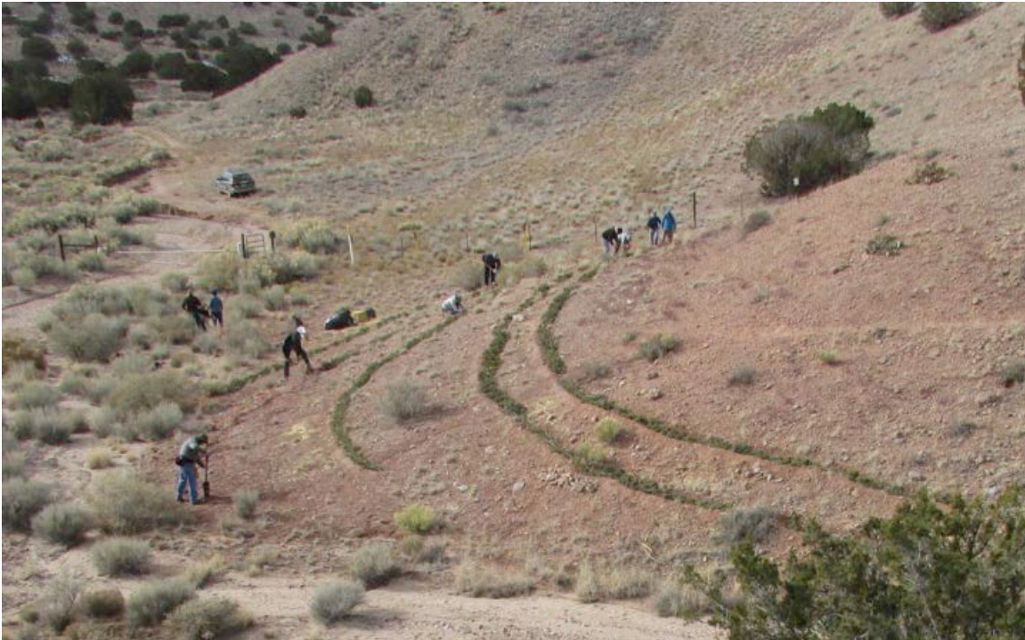
g. First series of berms in progress on first slope treated in the project.
